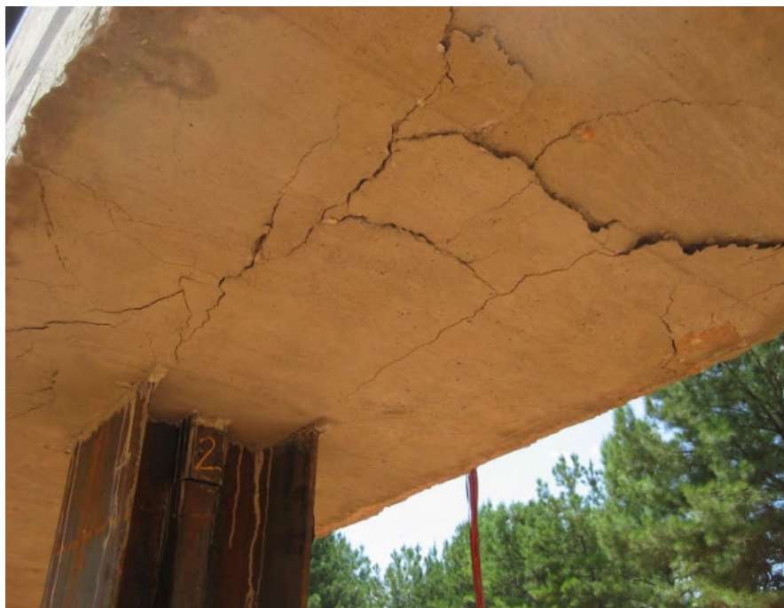
Figure 2-1: Flexural cracking of the bent cap (Marshall et al. 2017).
