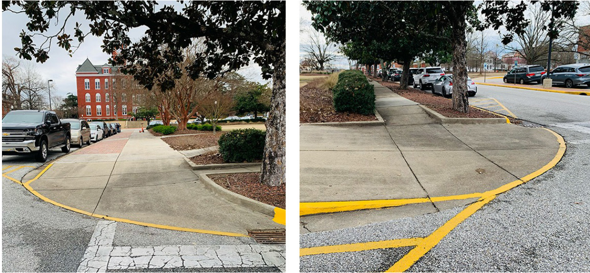
Figure 2.1: Sidewalk ramp accessibility.
