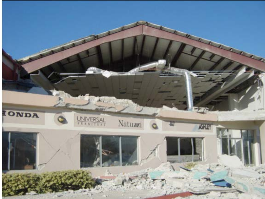
Figure 2.12. Infill Masonry Wall Collapse of PEMB in Port-au-Prince (Eberhard et. al. 2010)
