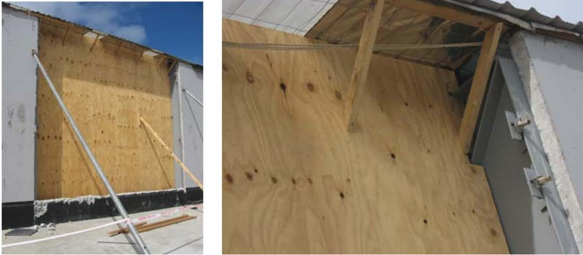
Figure 2.13. Loss of panel and temporary shoring of adjacent panel (Marshall and Gould 2012)
