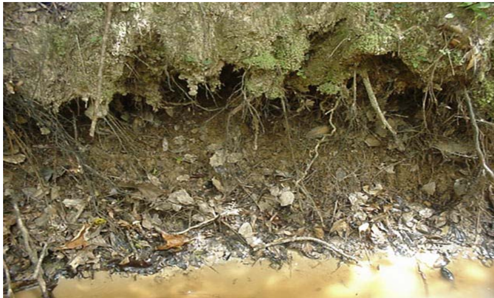
Figure 2.4 Channel scour on the bank of second-order stream (C3) during the pre-harvest period, September 9, 2004. (Source: Texas Forest Service)
