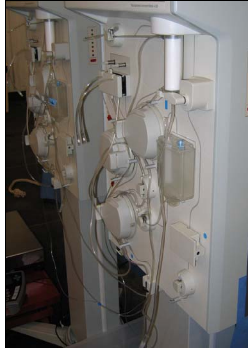
Separation device and reservoir properly installed
