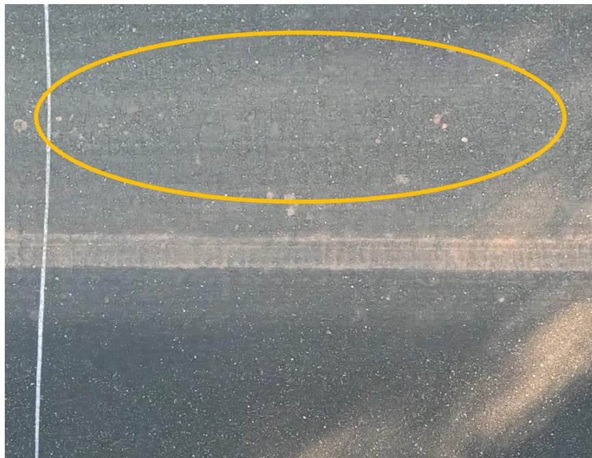
Figure 34. Initial Cracking on Off-Ramp Section with CR Surface Course
