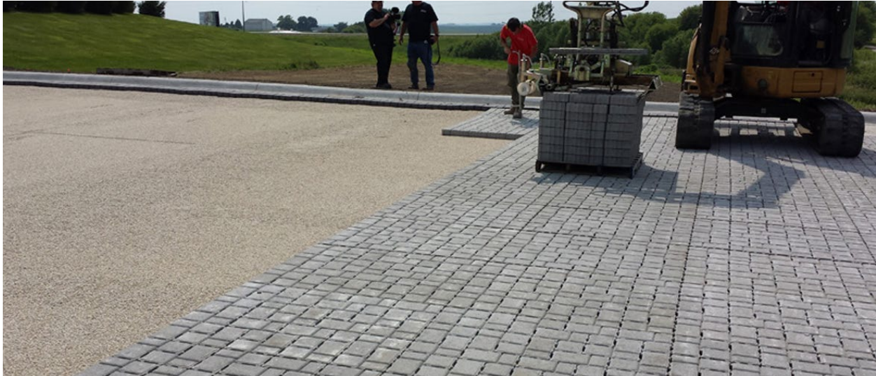
Figure 2.5: Permeable Pavers Parking Lot (US EPA 2022)
