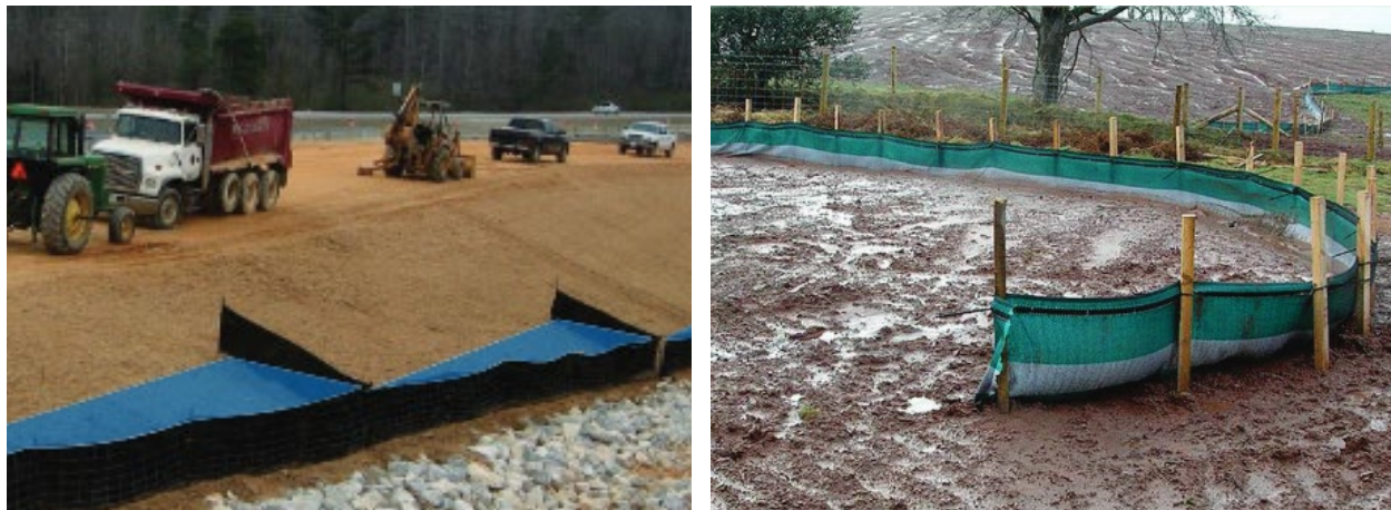
(a) silt fence J-hooks
