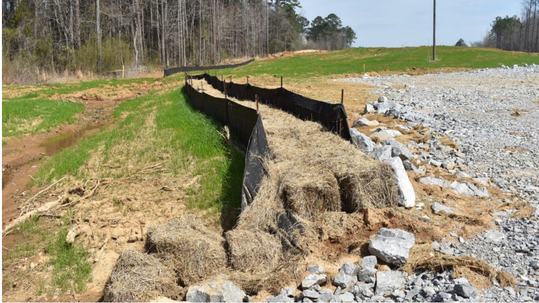
Figure 3.5: Sediment Retention Barrier (Perez 2016)
