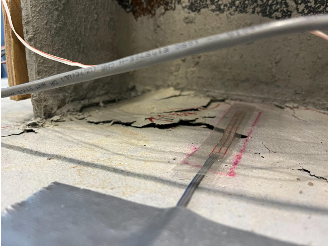
Figure 159. Specimen W-12-6 after final load stage (approx. 10 kips). Observed concrete crushing on the leading side.
