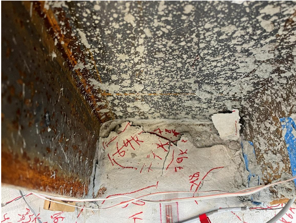
Figure 139. Specimen W-10-5 concrete crushing on leading side after target load of 8 kips (applied load of 6.2 kips) (load direction: from right to left).
