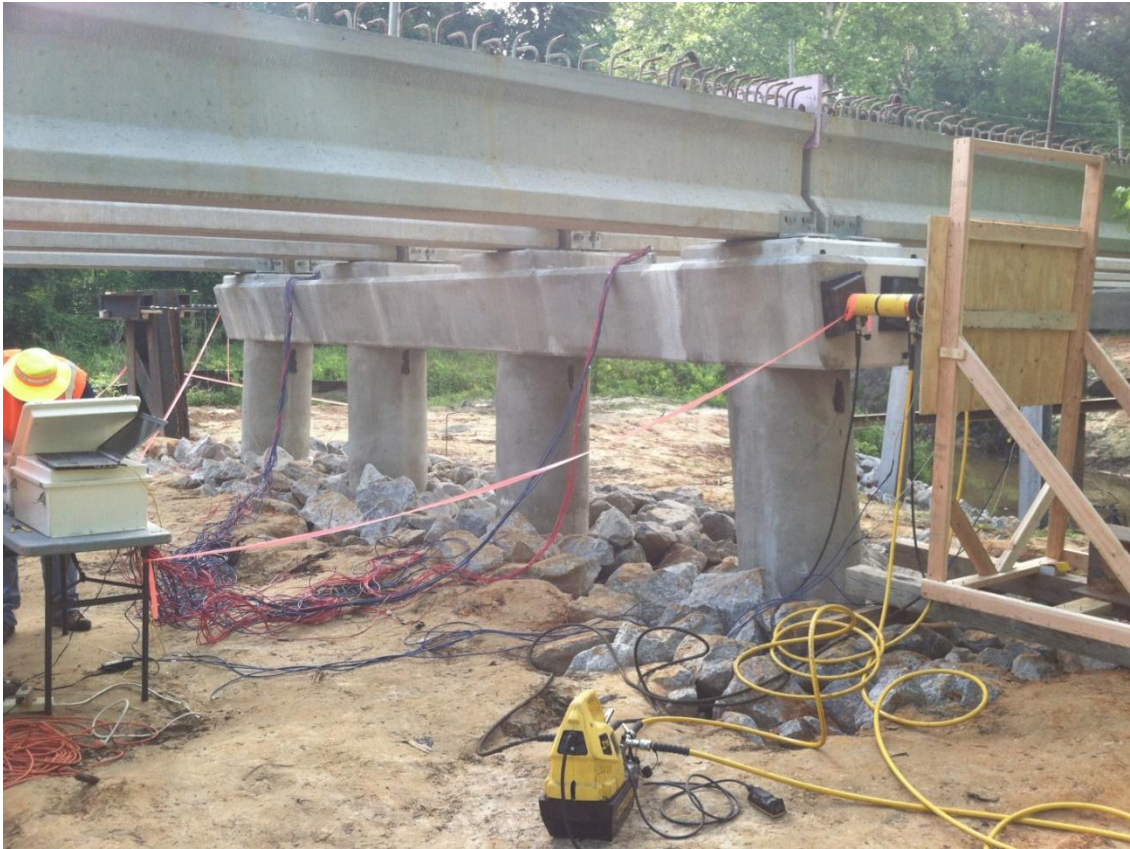
Figure 62. Field test setup on bridge over Old Town Creek, Alabama County Road 9, Macon County (Shorter, AL) (Marshall et al, 2017).
