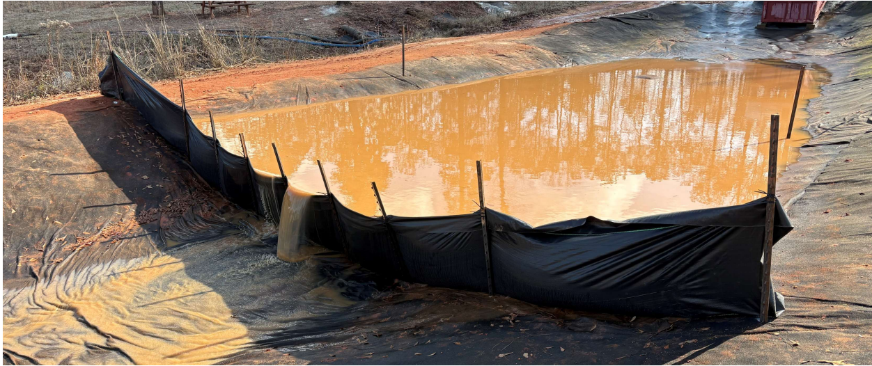
Figure 4.28: Installation 5 After Test C
