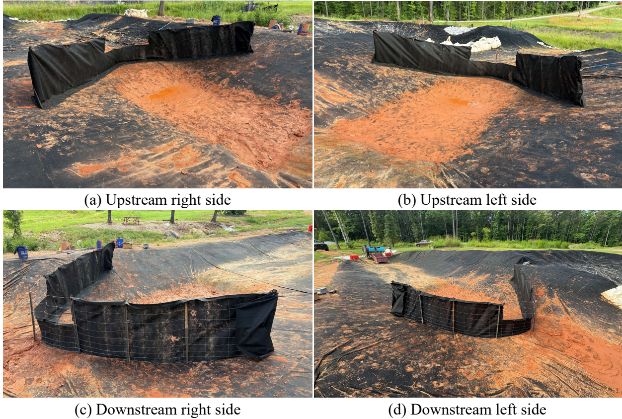
Figure 4.4: Modified Silt Fence
