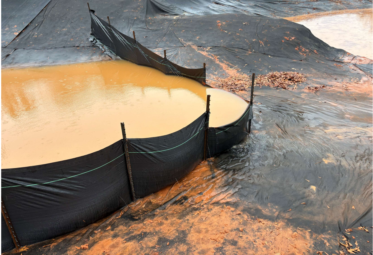
Figure 4.25: Installation 3 After Test C
