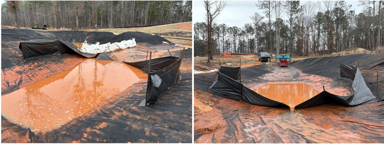
(a) Failure, facing downstream
